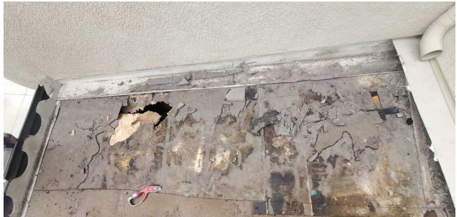
This section of roof was discovered to be leaking in November. The disintegration of the weatherproofing underlayment and holes in the plywood roofing indicate that the leaks had been occurring for years. An owner's garage had to have significant drying and mold remediation in the garage and soffit areas to mitigate the damage. This type of leak was not visible during annual maintenance inspections of the building roofs.
